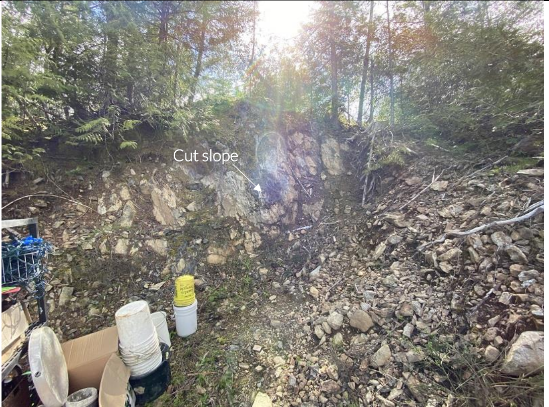
Photo 4: View of cut slope which exposed bedrock and overburden soils. Photo taken facing west.
